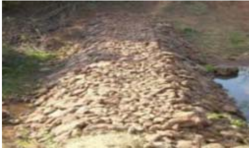
Figure 6: Loose Boulder structure
