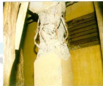
Figure 1a: Damage to columns in Himgiri apartment
