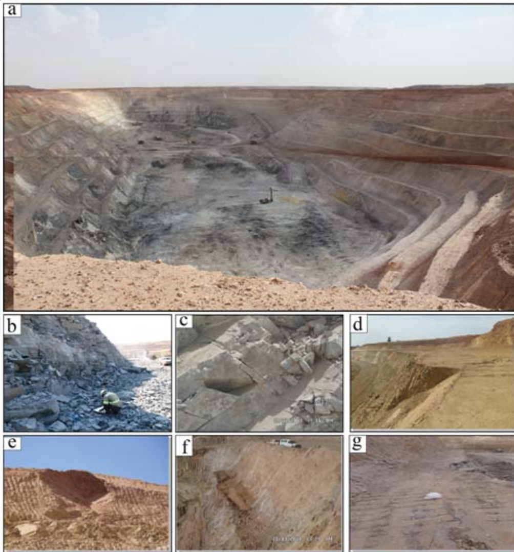
Photo: (a) Shooting of the northern pit of Inata gold mine, (b) Geotechnical mapping session, (c) Joints of varied orientations, (d) Planar failure on the wall; (e) Corner failure on the intersection of two joints of different orientations; (f) Area of the wall where the sizing of the bleachers and slope are not respected: the step width <math>< 5\text{ m}</math> and slope angle is
