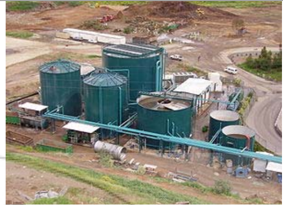
Figure 2: Two-stage, low solids, UASB digestion component of a mechanical biological treatment system near Tel Aviv
