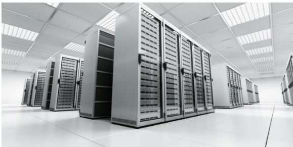
Figure 3: Servers at a data center
