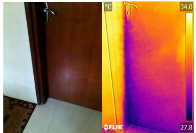
Figure 8: Air leakage through Meeting room
