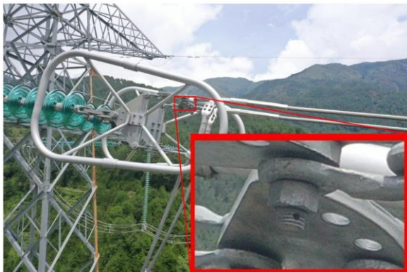
Figure 8: An annotated UAV image including defective bolts
