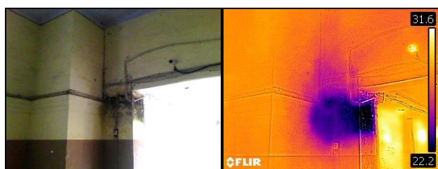
Figure 6: Infrared Detection of Leakage on wall from Damaged Plumbing Joint near Structural Department
