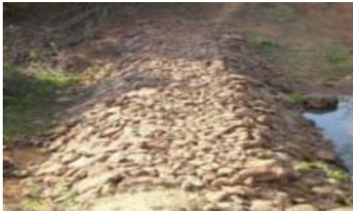
Figure 6: Loose Boulder structure
