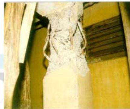
Figure 1a: Damage to columns in Himgiri apartment
