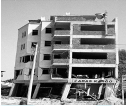
Figure 1b: Soft story failure, Bhuj 2001
