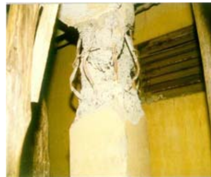
Figure 1a: Damage to columns in Himgiri apartment
