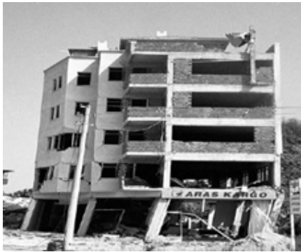
Figure 1b: Soft story failure, Bhuj 2001
