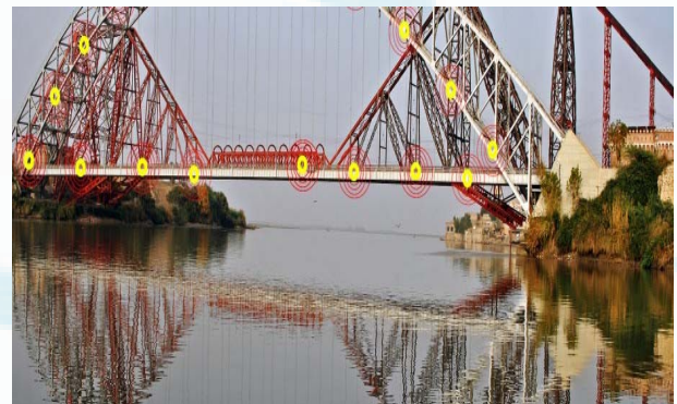
Figure 1: Structural Health Monitoring with sensors on a Bridge
