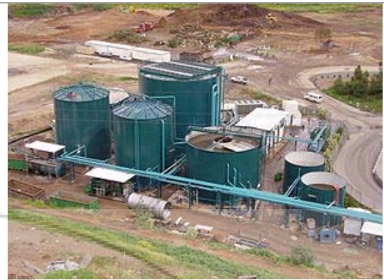
Figure 2: Two-stage, low solids, UASB digestion component of a mechanical biological treatment system near Tel Aviv
