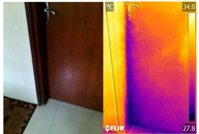
Figure 8: Air leakage through Meeting room
