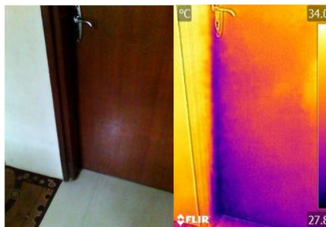
Figure 8: Air leakage through Meeting room
