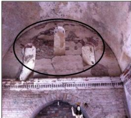
Figure 3 (a): cracks on the walls of the St. Matthias
